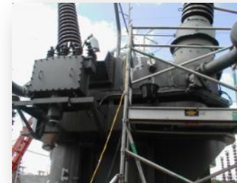
Acoustic sensors (70-250kHz) tested in Northfleet 400kV transformer
